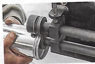
03] After mocking up the new duct and cutting off the legs to the correct length, Sanchez says, "I rolled each end of the ducts on my bead-roller so everything seals up tight. You can buy reasonably efficient and priced bead-rollers from Eastwood or Harbor Freight."
